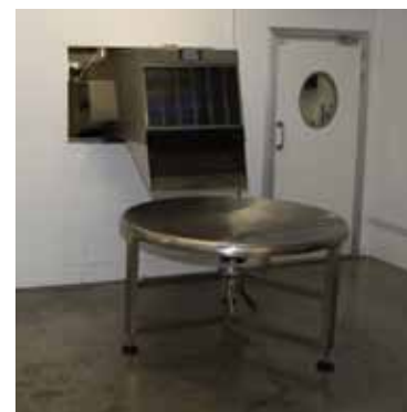
Outlet for discharging bags onto rotary table
